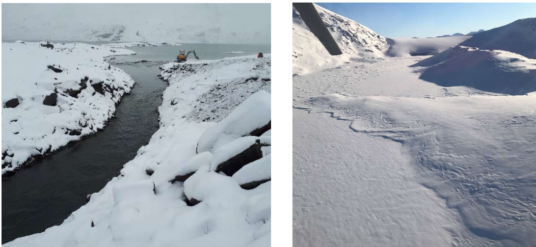
Figure 14-6 The finished drainage channel looking towards Nordvatnet in October 2017 (left). Nordvatnet in March 2018 looking towards the glacier (right). Photos: Leif Martin Hansen and Miriam Jackson.
