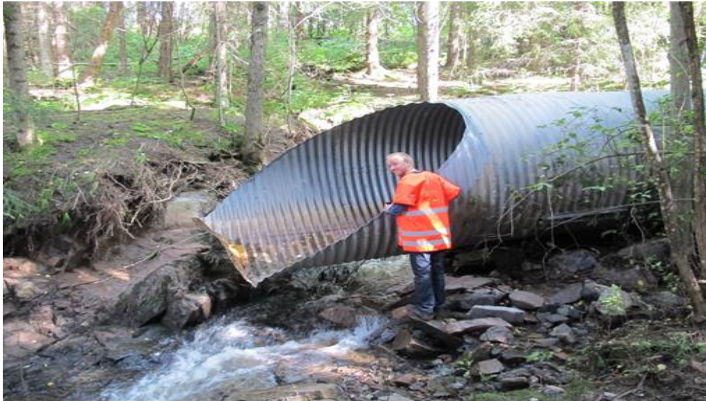
Photo: Culvert gone astray after local flooding in Buskerud (20121806, Andreas Gjærum – NPRA)
