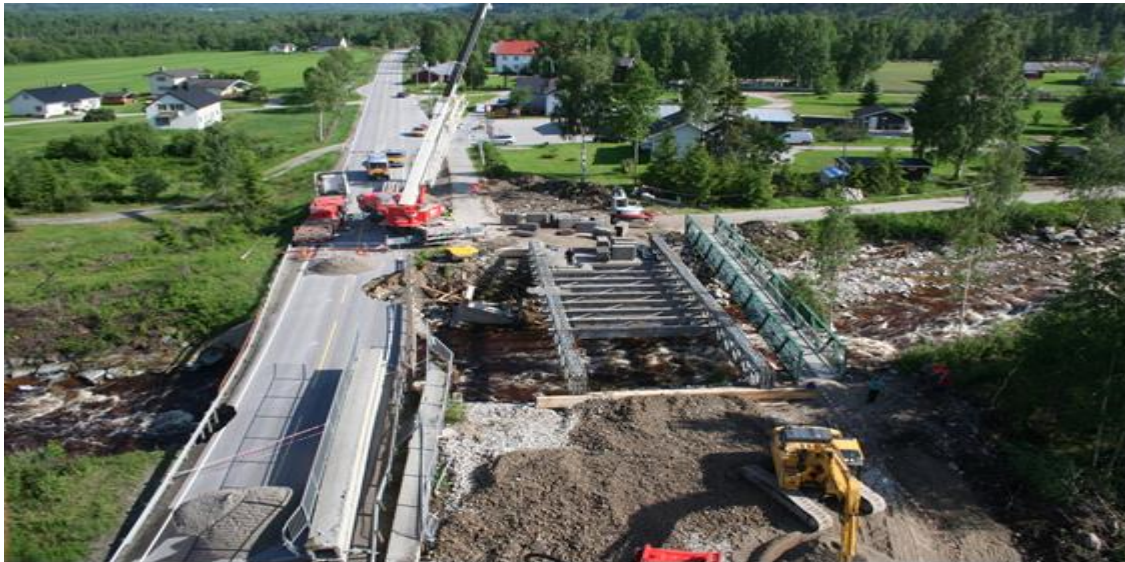
Photo: Trya Bridge on National Highway 3 after the floods at Whitsun in the valley of Østerdalen (2011 - NPRA)
