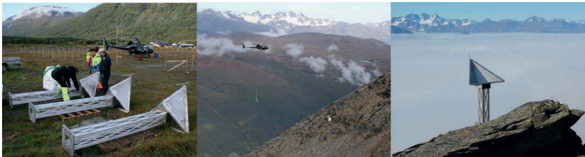
Figure 10: Overview of installation of a corner reflector in Troms County. The reflectors provide stable signal, and are covered to prevent snow accumulation.
