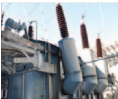
300/132 kV transformator. Foto: Henning Weyergang-Nielsen, NVE
