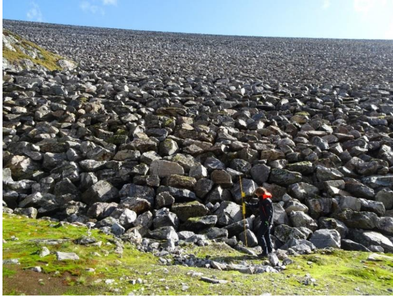
Figure 2. Placed riprap constructed on the downstream slope of dam Oddatjørn, which is a 142 m high rockfill dam constructed in Suldal, Norway (Photo: GHR Ravindra, NTNU).
