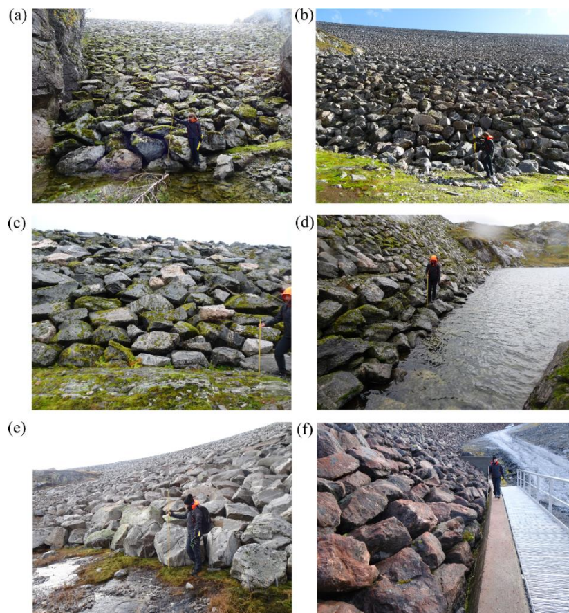
Figure 12. Depiction of existing conditions of placed riprap toe sections. Category 1 at dams (a) Fjellhaugvatn dam (b) Oddatjørn dam and (c) Skjerjevatnet main dam. Category 2 at (d) Skjerjevatnet main dam. Category 4 at (e) Storvass dam. Category 5 at (f) Akersvass dam (Adopted from Ravindra et al., 2019a).
