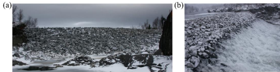
Figure 16. (a) Image of the test rockfill embankment (M1) from the test site downstream of Røssvatn, southern Norway prior to testing; (b) Image of the test dam during testing (Image courtesy: EBL Kompetanse (2006) and published in Ravindra et al., 2019b).
